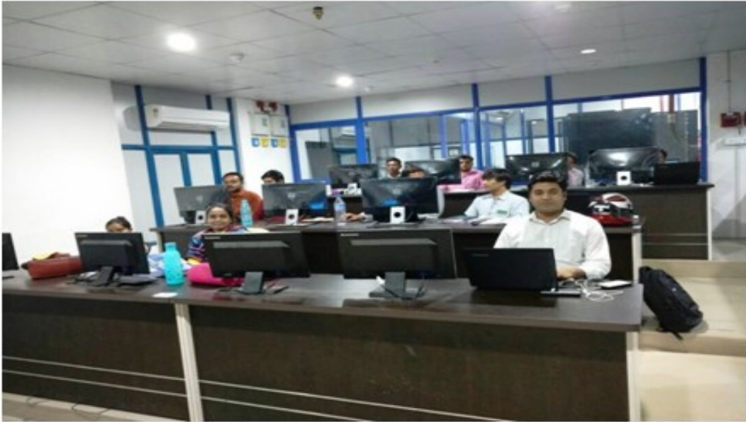
ITMS Control Room
